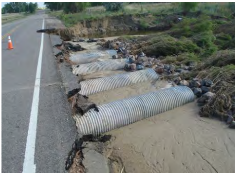
Plugged culverts at Picadilly Ave. and Coal Creek
