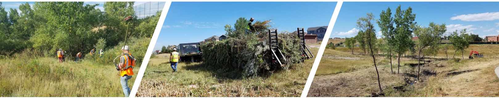
LEFT: Unnamed Creek prior to vegetation removal. MIDDLE: Over 1 million pounds of vegetation recycled. RIGHT: The resulting 'clear zone' for Unnamed Creek.
