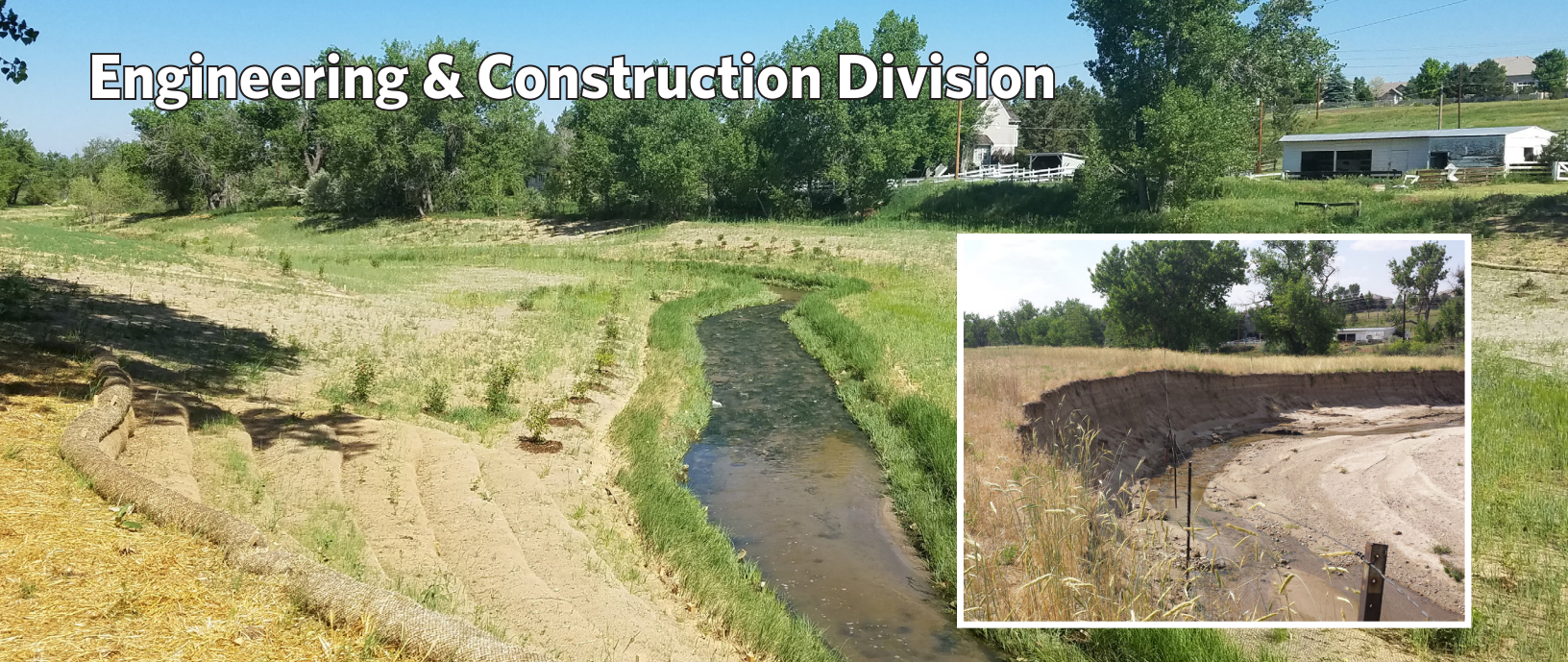
Redefinition of the Piney Creek channel through the Ranches development results in a stable channel and bank with a decrease in sediment transport downstream.
